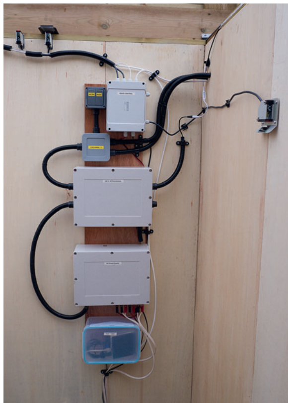
fig.9 The electrical systems are mounted in waterproof containers onto a plywood panel. From the top; power switches, Arduino controller, mains junction box, mains distribution box, DC power supplies and the NUC sits in a sealed food container at the bottom for easy access along with its external solid state drive. The three reflective sensors, two for the roof and one for the mount are mounted to the walls. Illumination is provided by an IP65 LED strip around the top of three walls.
