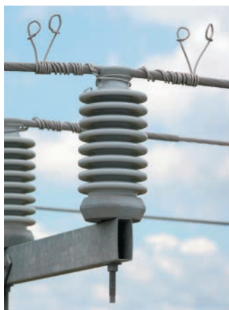
▲ Ceramic electrical insulator
